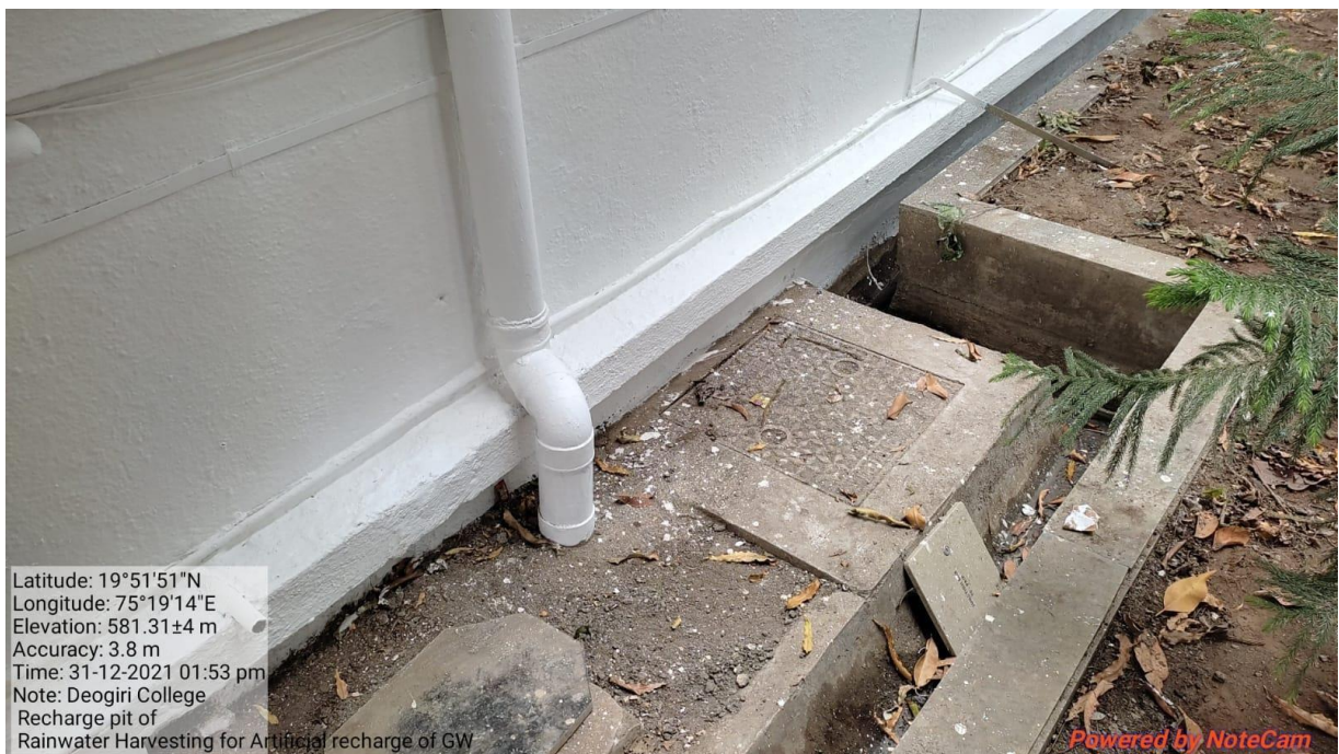
Fig 8:- Roof water harvesting of College building for artificial recharge of bore well / dug well
