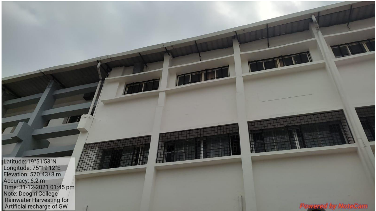
Fig 11:- Roof water harvesting of College building for artificial recharge of bore well / dug well
