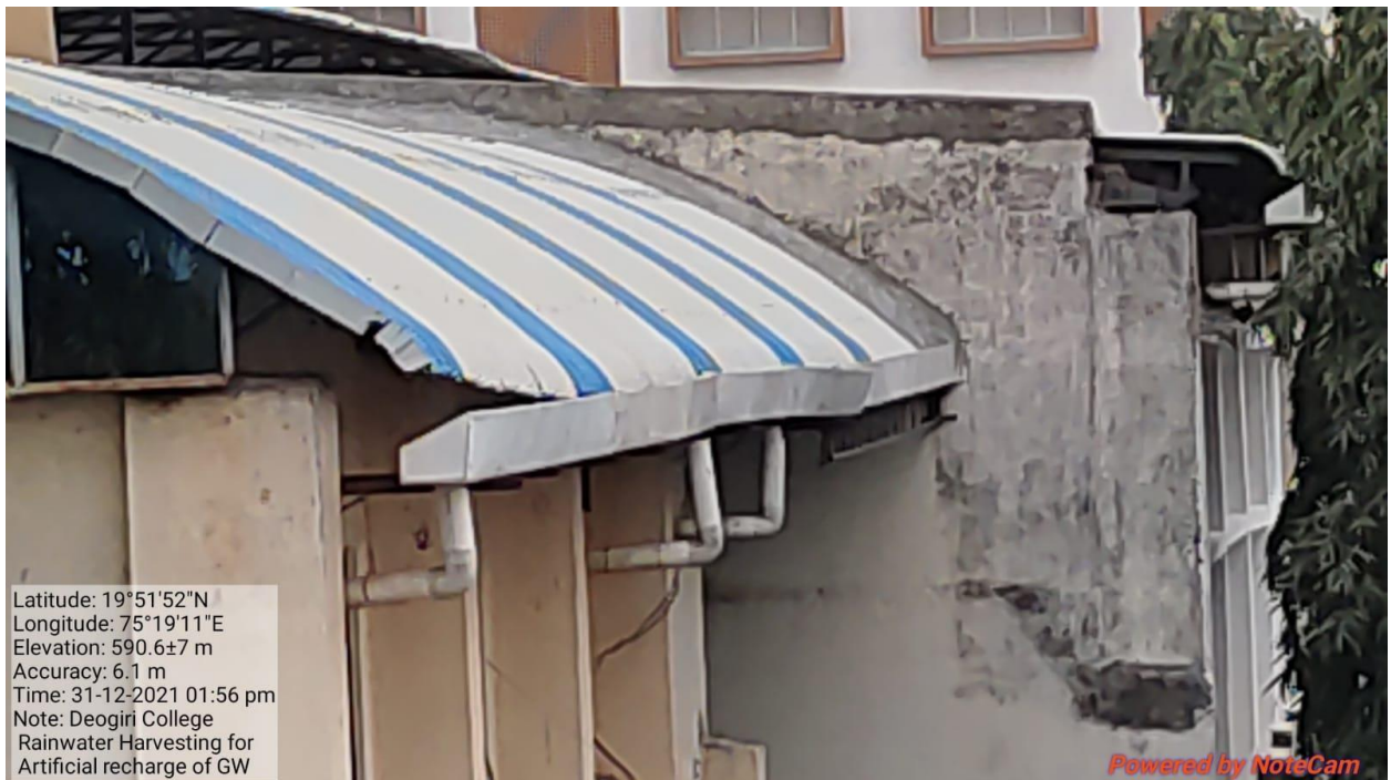
Fig 5:- Roof water harvesting of College building for artificial recharge of bore well / dug well
