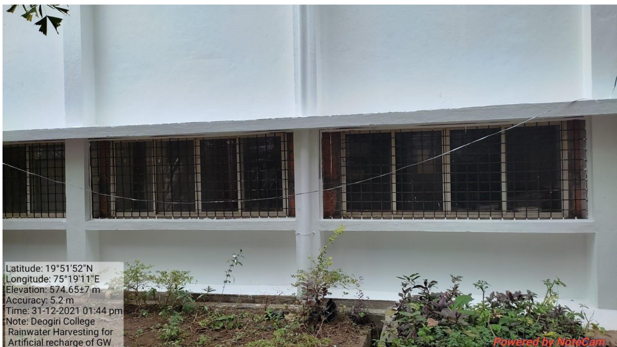
Fig 6:- Roof water harvesting of College building for artificial recharge of bore well / dug well
