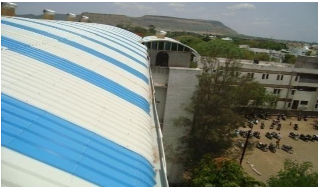
Fig 4:- Roof water harvesting of College building for artificial recharge of bore well / dug well
