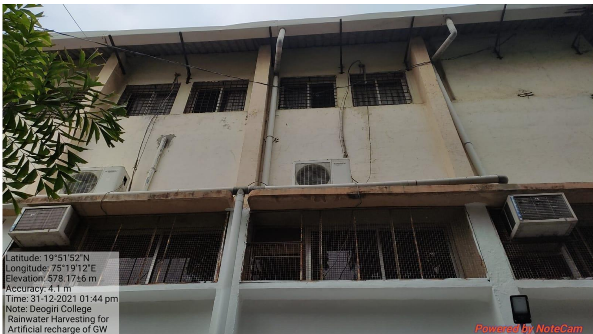
Fig 12:- Roof water harvesting of College building for artificial recharge of bore well / dug well
