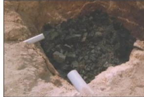
Recharge Pit of 5 x 5 x 7 feet near borewell
