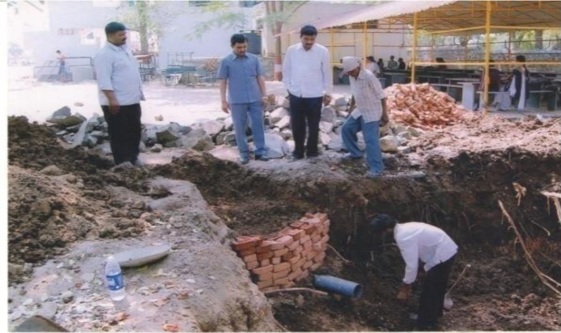
Fig 1:- Recharge Filter bed (15x15x10)near Dug Well
