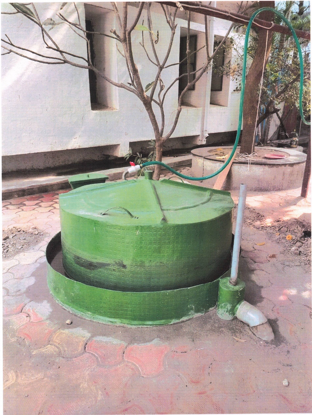
Biogas Plant installed at Girl's hostel, Deogiri College, Aurangabad.
