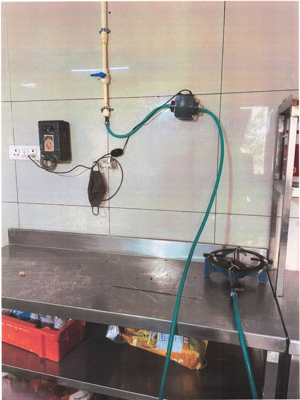
Biogas connected to girl's hostel mess kitchen
