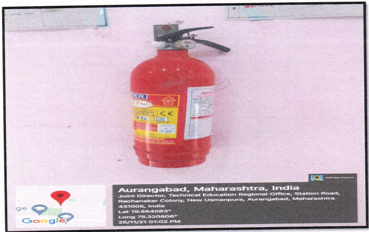
At Biotechnology Lab First Floor
