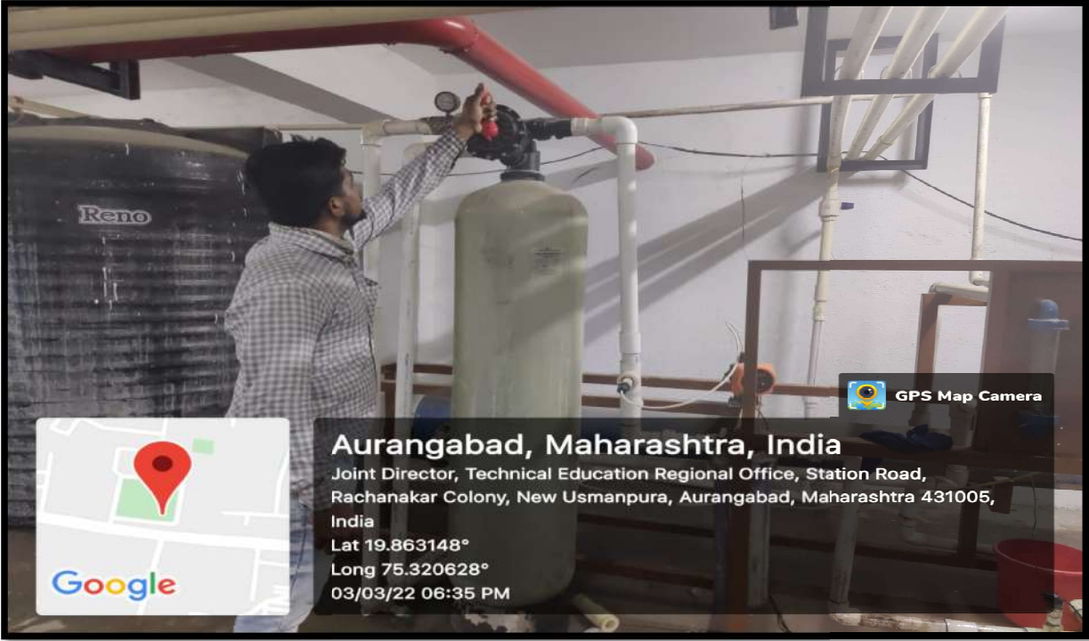
Fig 1:- Maintenance of RO water filter
