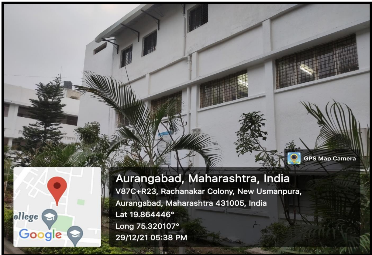
Fig. 06 and 07 - Rainwater Conduit Pipelines on College building
