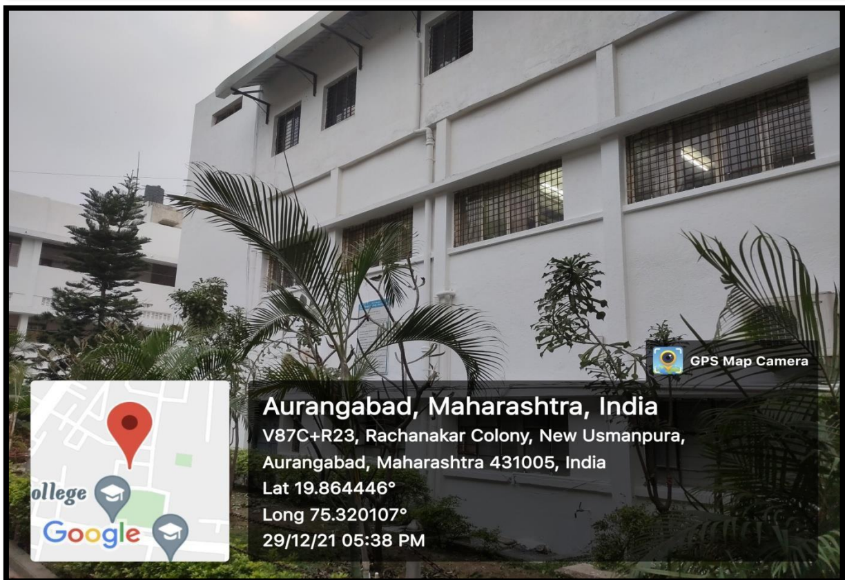
Fig. 09 and 10 - Rainwater Conduit Pipelines on College building
