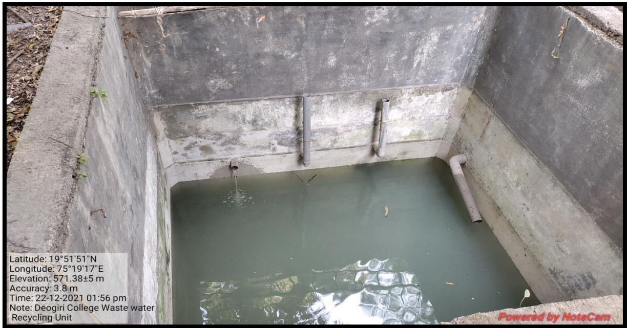
Fig 04:- Final sediments trap pit of Water recycling unit.
